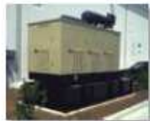
AC/DC Site Generation
