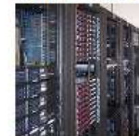
Data & Telecom Centers
