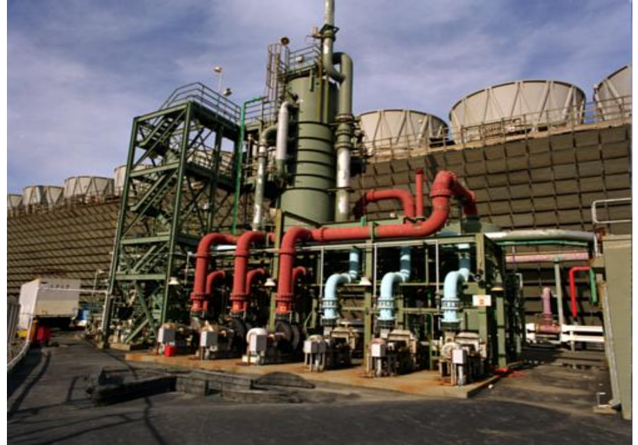
Condensers and cooling towers, The Geysers, being fitted with direct contact condensers developed at NREL
